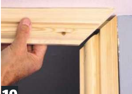
19 Cramp vertical architrave in position and check fit of top piece. Trim mitres if necessary with block plane
